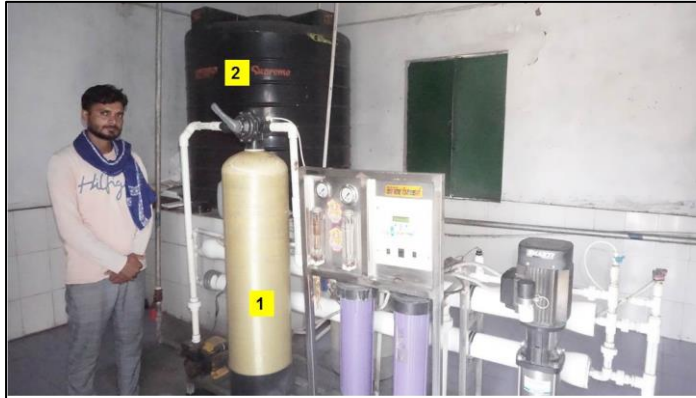
1. R.O. Plant. 2. Processed Water Storage Tank (2KL).
