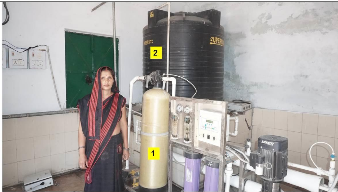
1. R.O. Plant. 2. Processed Water Storage Tank (2KL).
