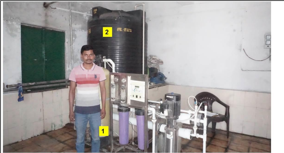
1. R.O. Plant. 2. Processed Water Storage Tank (2KL).
