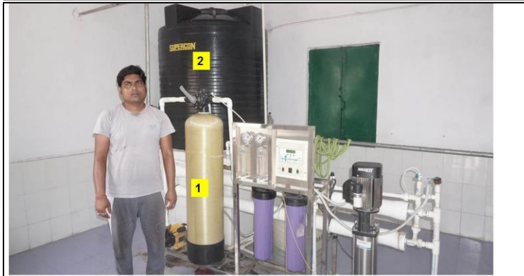
1. R.O. Plant. 2. Processed Water Storage Tank (2KL).
