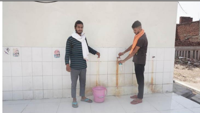
Outlet of Purified Water
